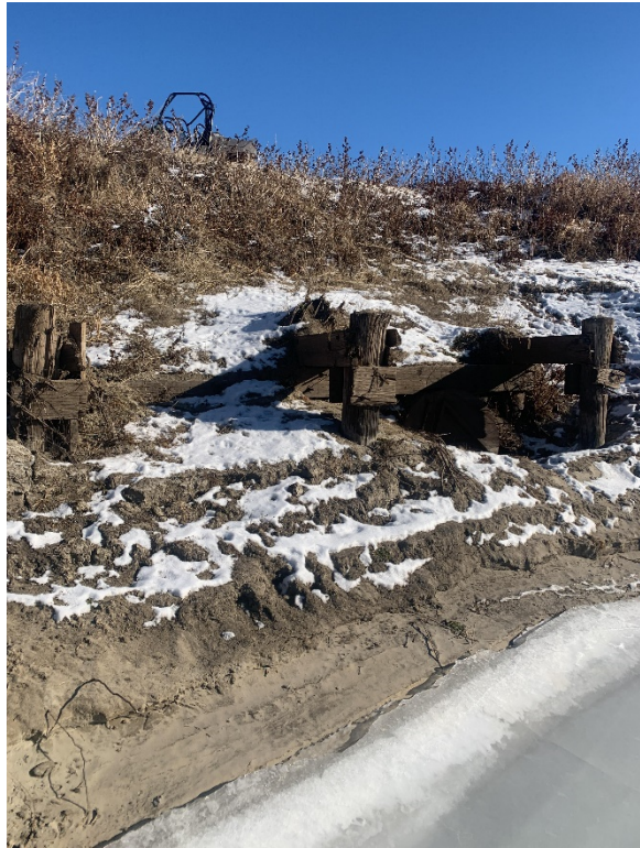
Figure 3: Pipe silted shut
