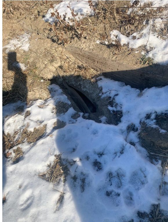
Figure 2: Pipe silted shut (side view)
