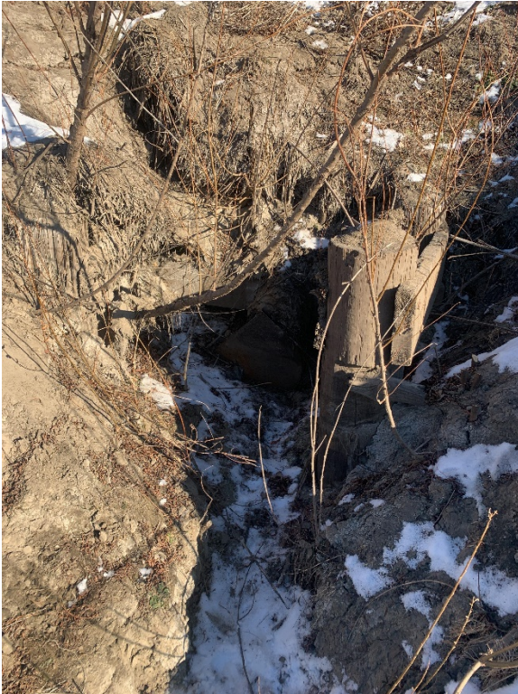
Figure 1: Pipe silted shut (front)
