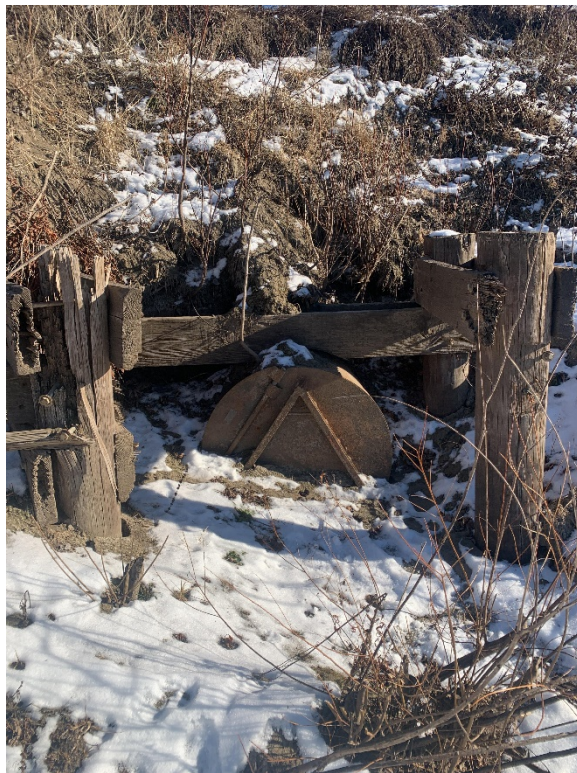
Figure 4: Pipe silted shut
