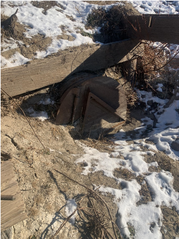
Figure 5: Pipe silted shut
