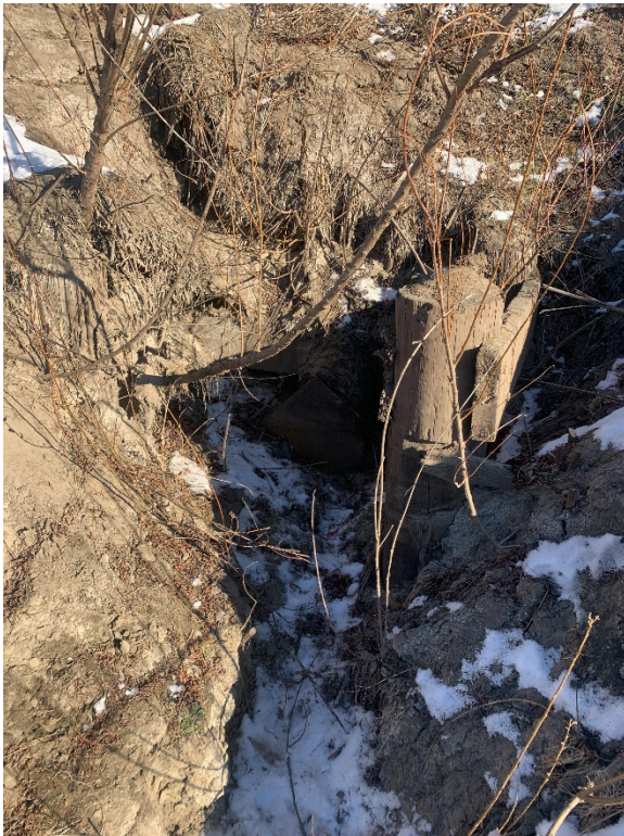
Figure 1: Pipe silted shut (front)
