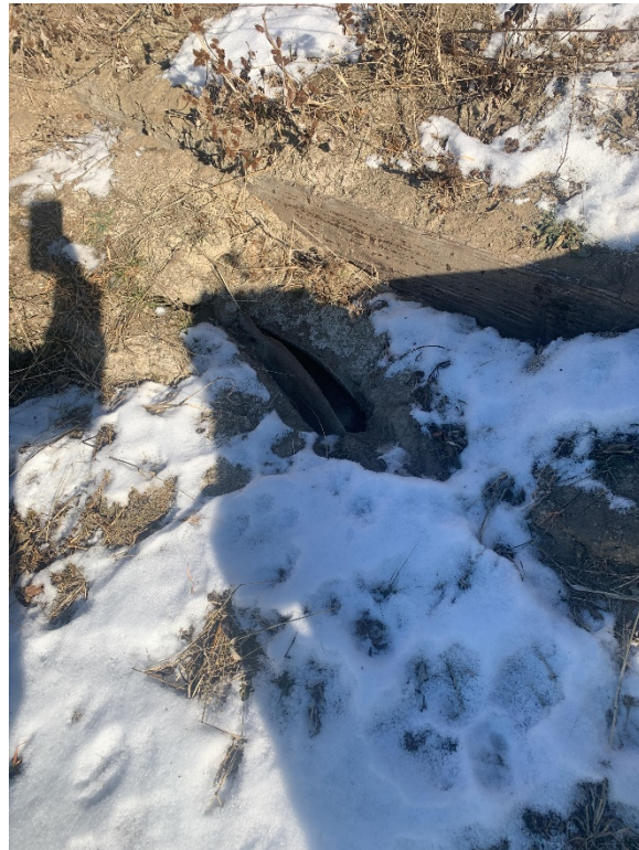
Figure 2: Pipe silted shut (side view)
